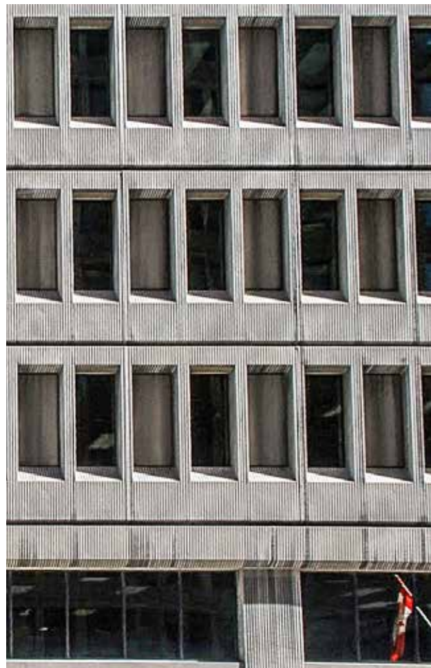
The Brutalist conversion currently on display at 360 Laurier Avenue West. ROBERT SMYTHE/THE BUZZ
