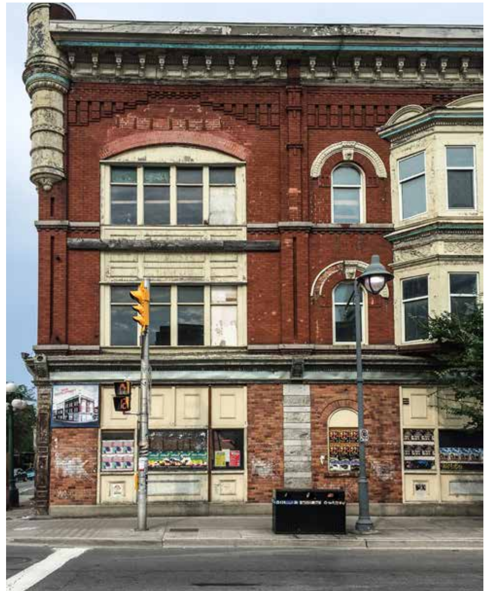
The dilapidated current state of Somerset House, at Bank and Somerset. ALAYNE MCGREGOR/THE BUZZ
