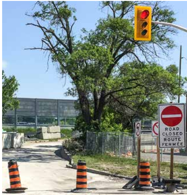
The Lyon on-ramp to the Queensway is closed for this year's work to replace the Bronson and Percy overpasses.
