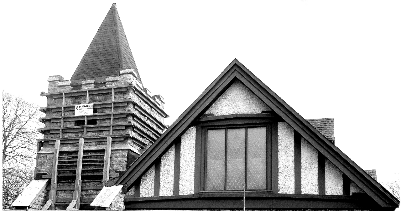
The tower of Eglise Unie St-Marc is now shored up pending repairs.
