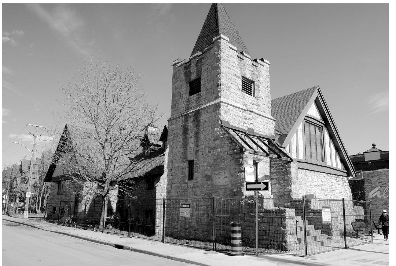
The church after cracks were discovered in the tower.
