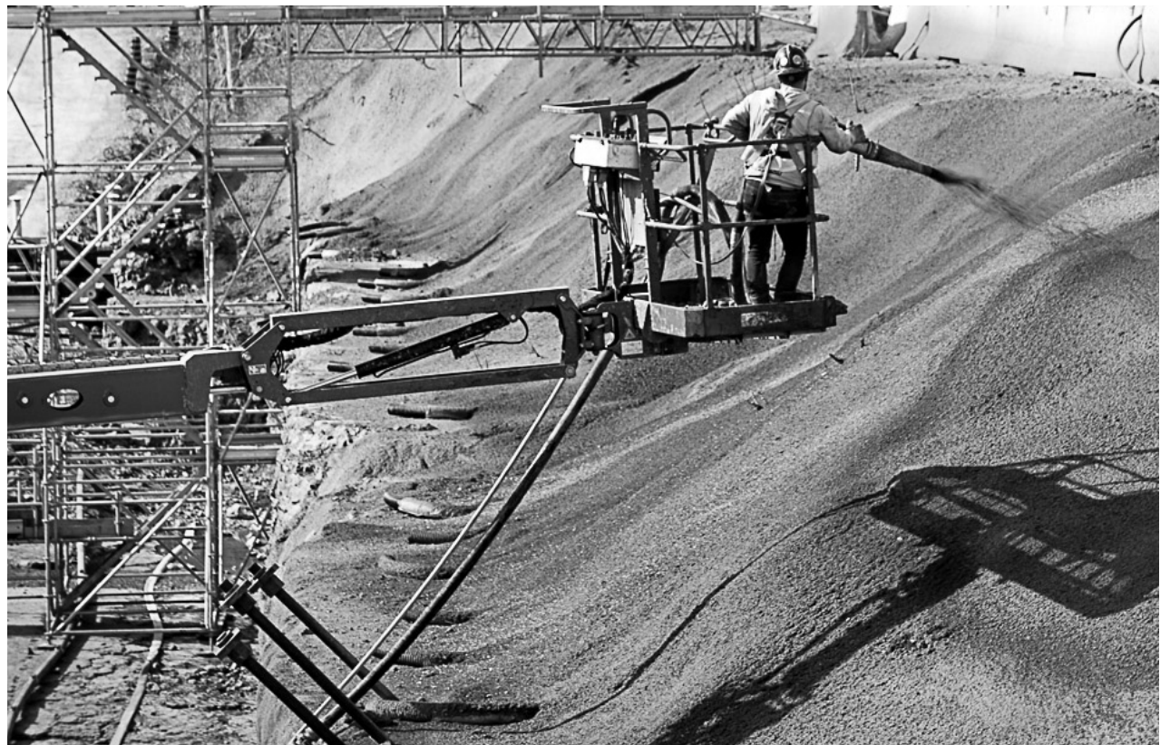
The new Corso Italia LRT station is currently under construction in the LRT Line 2 trench just north of Gladstone Avenue. Here, a worker applies anti-erosion spray. BRETT DELMAGE/THE BUZZ
